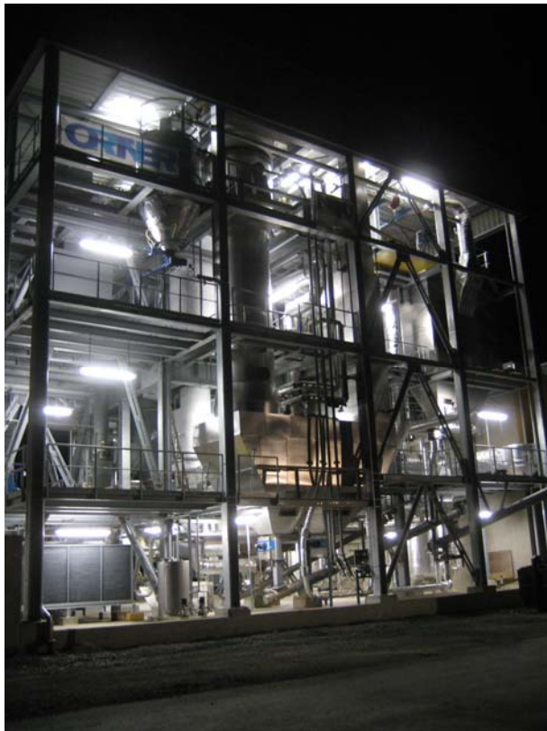
Figure 2: dual fluidised bed gasifier in Oberwart
